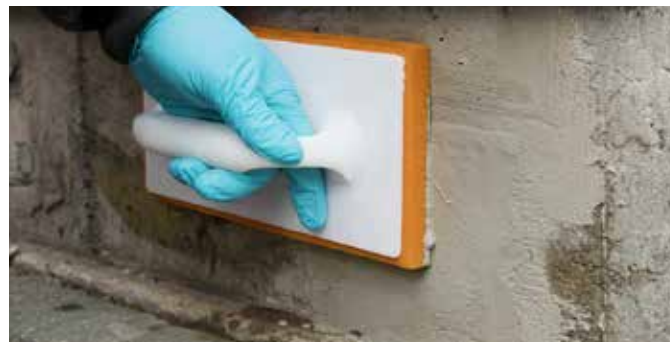
5 As soon as the setting begins, the surface can be smoothed with a trowel or float.
